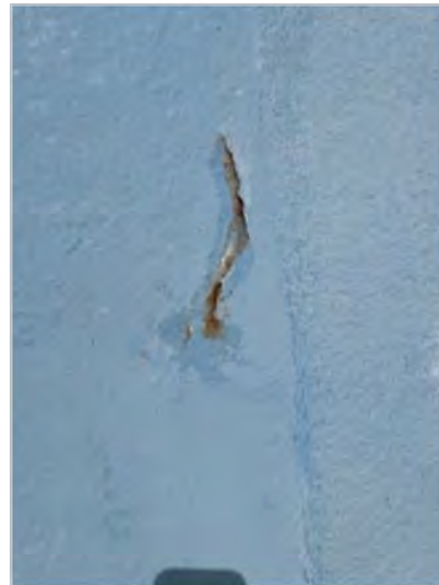
Crack in wall of main pool
