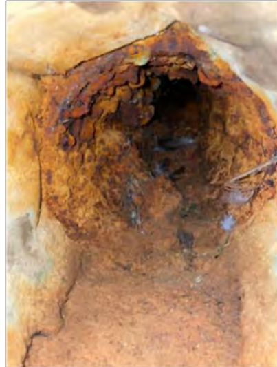
Deteriorated cast iron pipe
