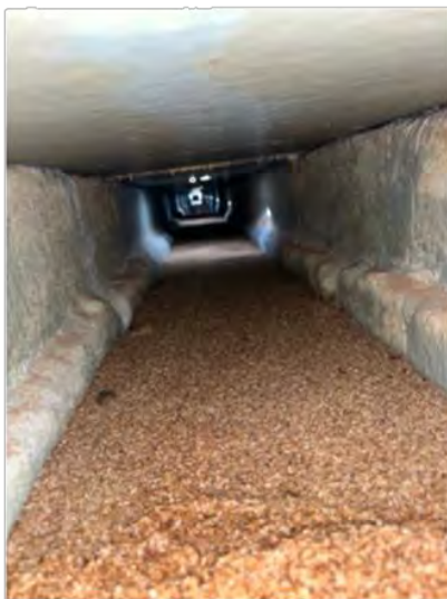
Blockage in pipework
