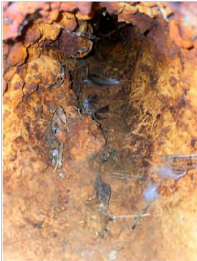
Deteriorated cast iron pipe
