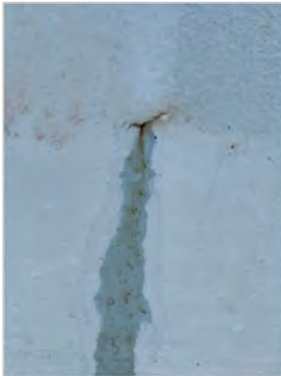
Crack in wall of main pool
