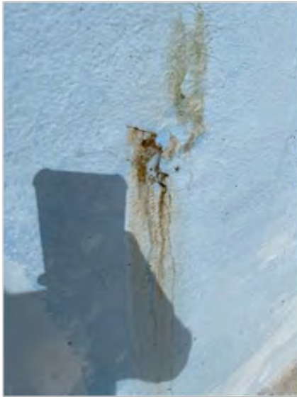
Crack in wall of main pool
