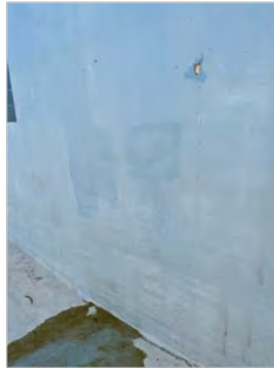
Crack in wall of main pool
