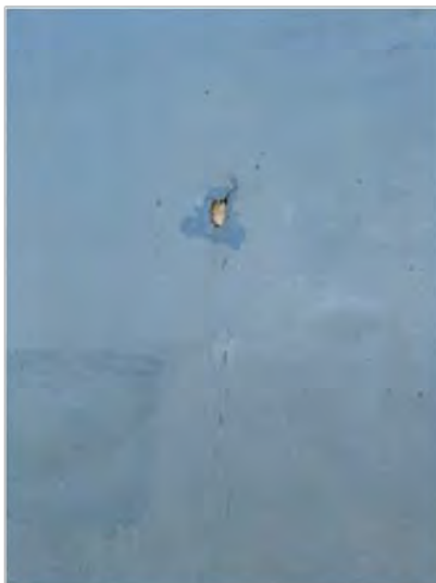
Crack in wall of main pool
