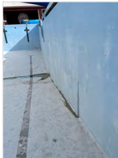
Crack in wall of main pool
